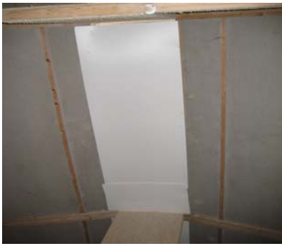
Figure 13. Vents sealed with lightweight plastic
